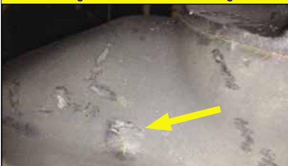
Bulge/crack in carrier housing
